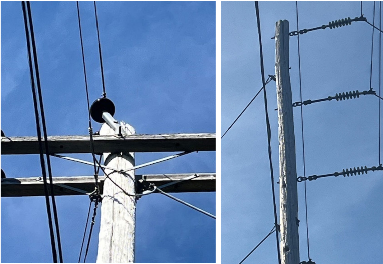
Figure 6 – Bent Insulator and Pole Damage on GLV-02
