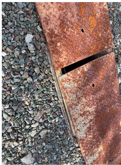
Figure A-10: BLK Cable Trench
