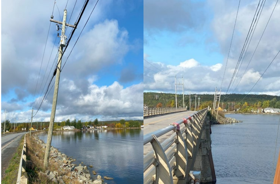
Figure 2 – Leaning Poles on Causeway Section
