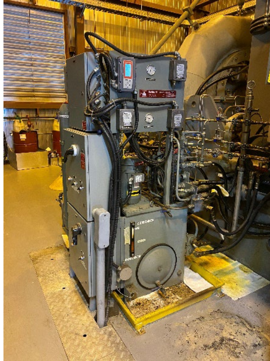
Figure 4 – Governor Hydraulic Power Unit
