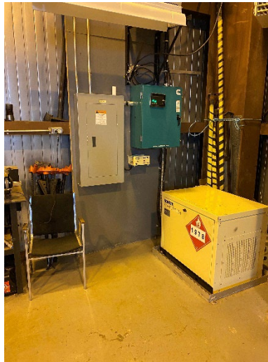
Figure 6 - Auxiliary Power Unit
