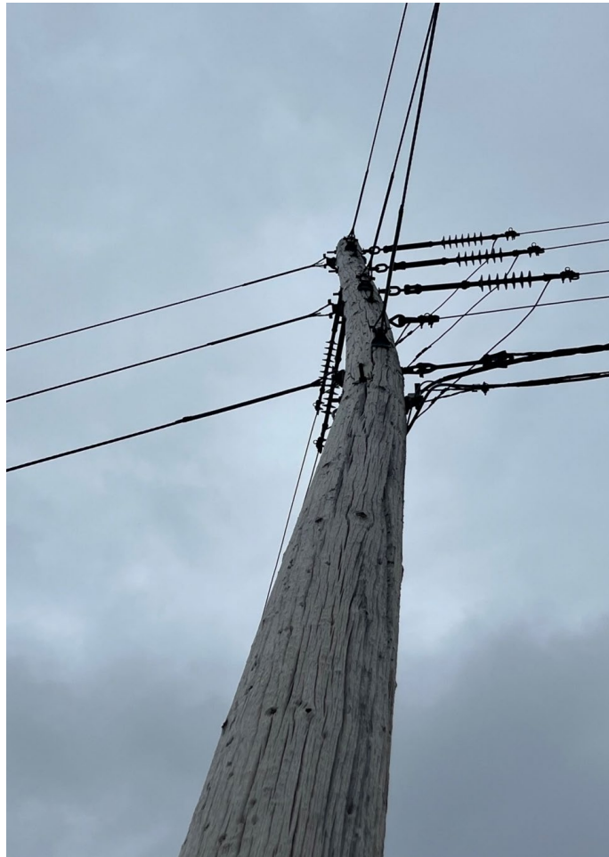
Figure 5 – Pole Along GLV-02 with Advanced Structural Degradation
