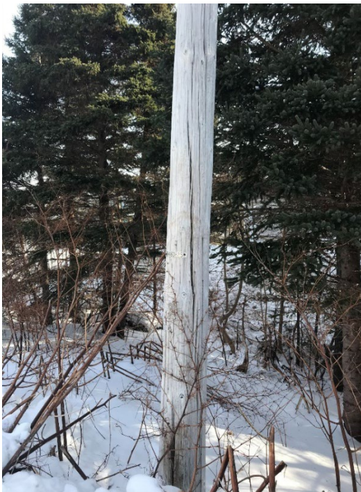
Figure 2 - Severe cracks in Feeder Trunk pole
