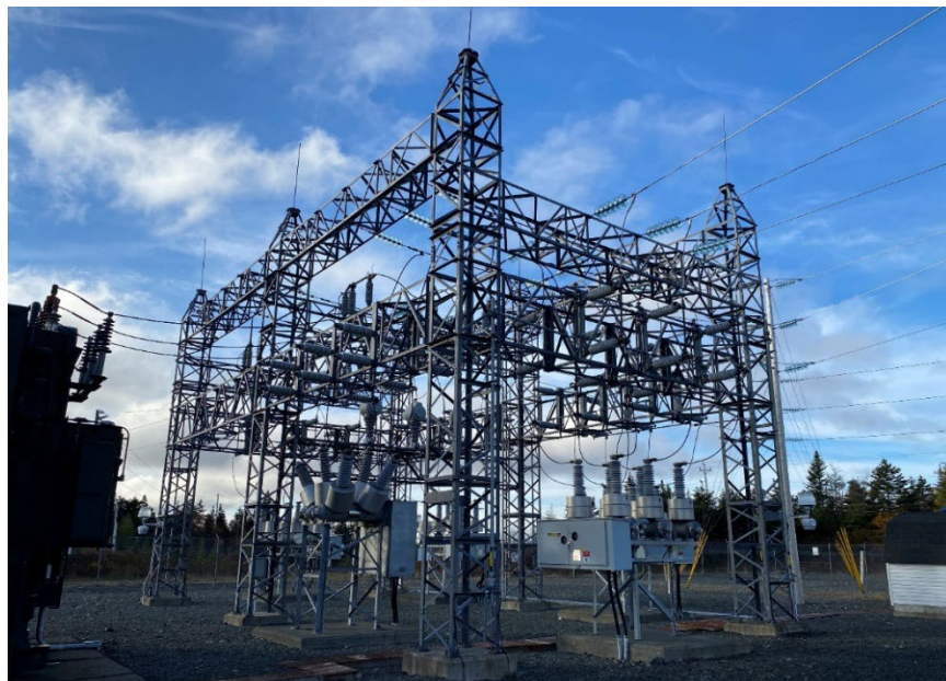
Figure A-2: BLK Substation
