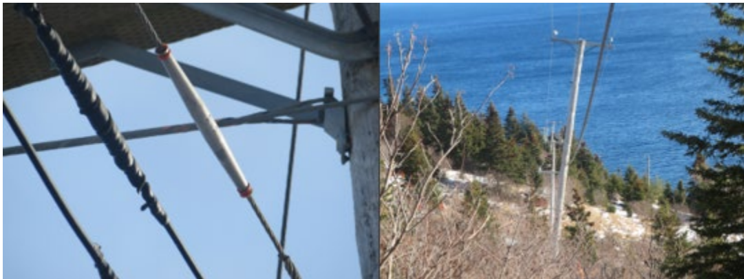
Figure 4 – Non-Standard Sleeve Repair (left) and Leaning Pole (right)
