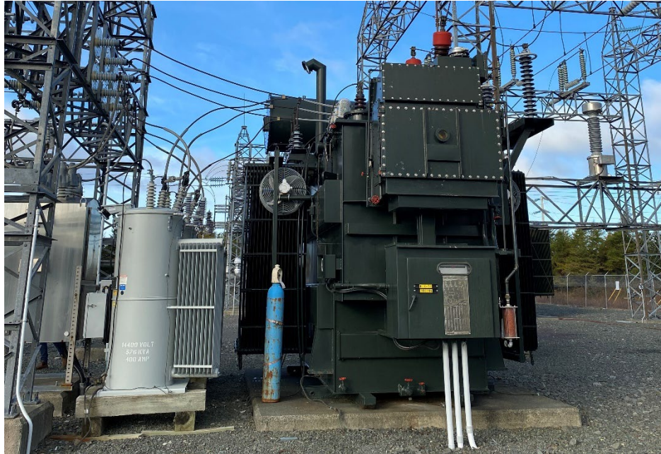
Figure A-5: BLK-T2 Power Transformer
