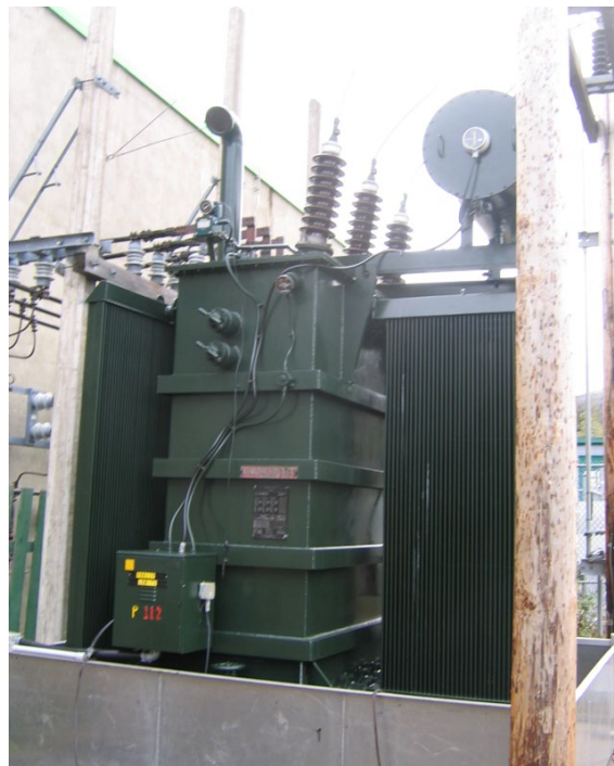
Figure B-1: Power Transformer LBK-T1.
