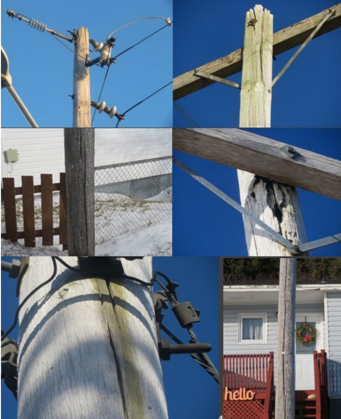
Figure 2 – Cracking and Deteriorated Poles
