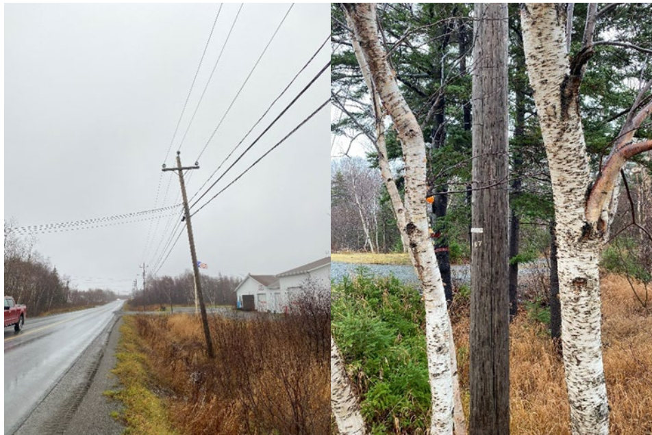
Figure 3 – Leaning and Deteriorated Poles
