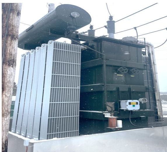
Figure C-3: Power Transformer MOP-T1
