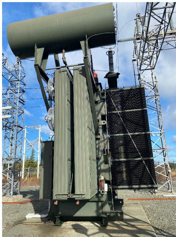
Figure A-4: BLK-T3 Power Transformer
