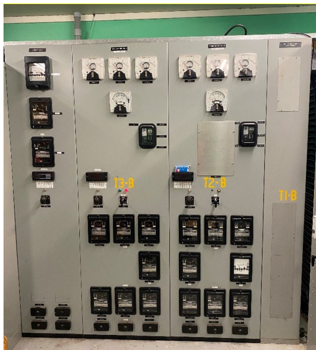
Figure A-6: Electromechanical Relays
