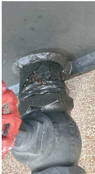
Figure A-4: 2025 inspection on valve
