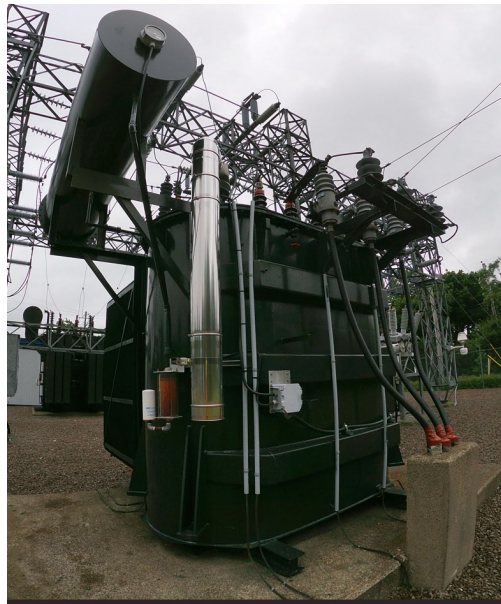
Figure D-1: Power Transformer RRD-T3
