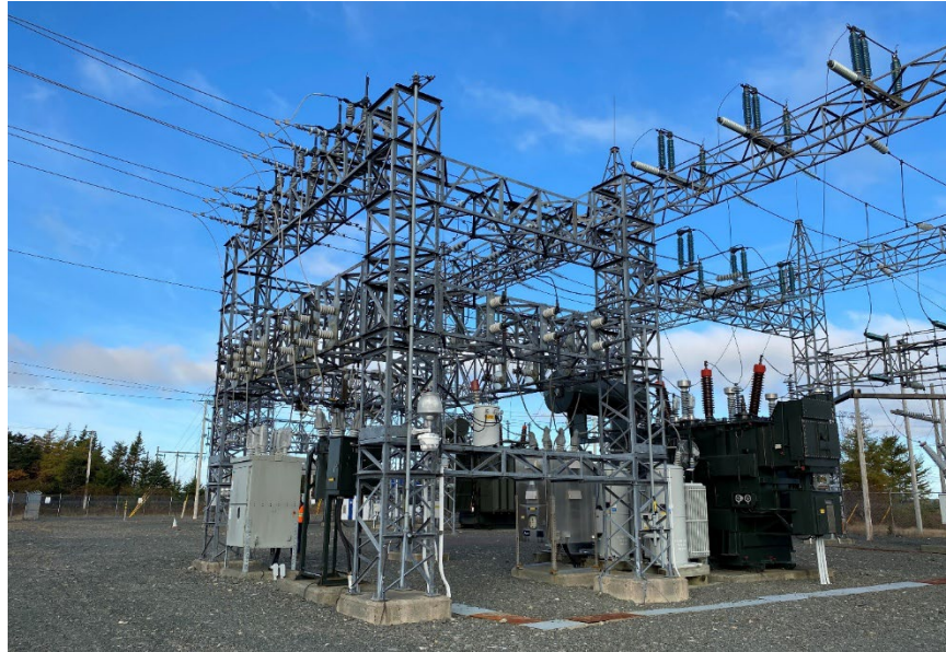
Figure A-1: BLK Substation
