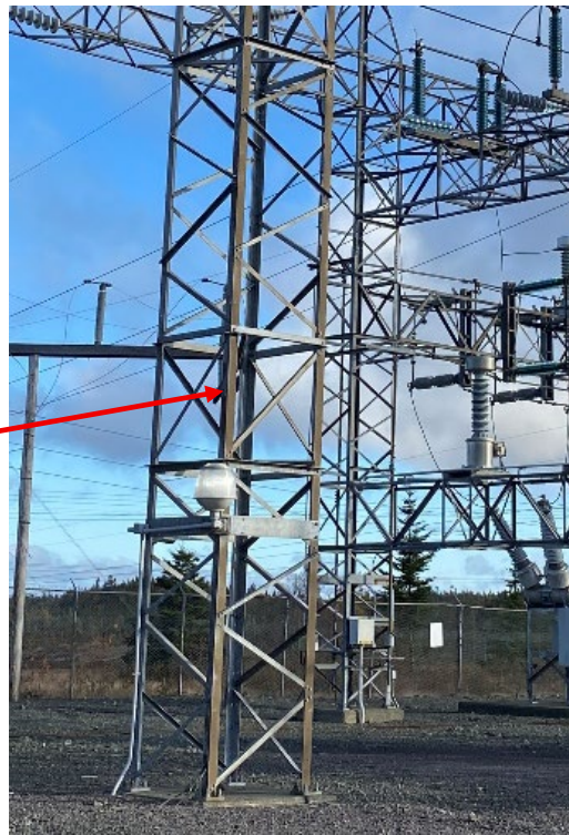
Figure A-3: 138 kV Structure Surface Corrosion
