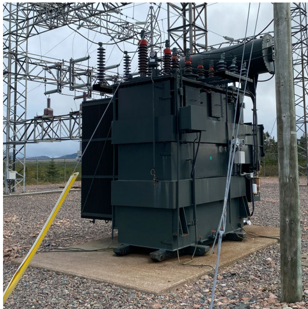
Figure A-1: Power Transformer LAU-T1
