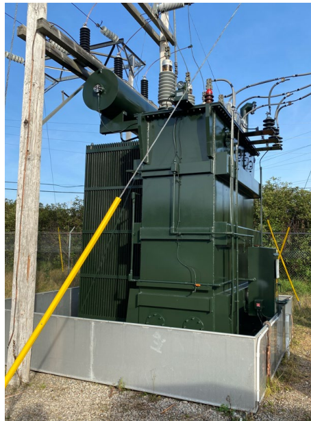
Figure C-1: Power Transformer HAR-T1.
