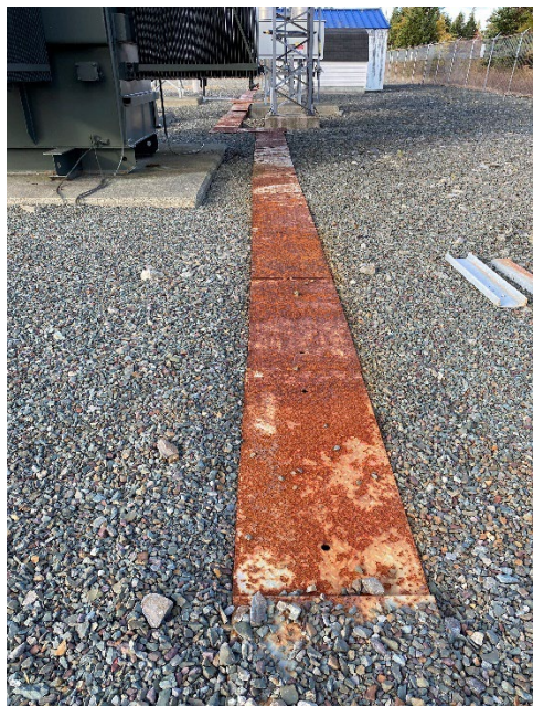
Figure A-9: BLK Cable Trench
