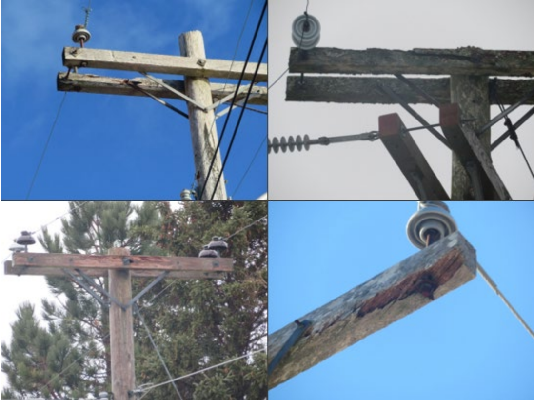
Figure 3 – Deteriorated Cross Arms
