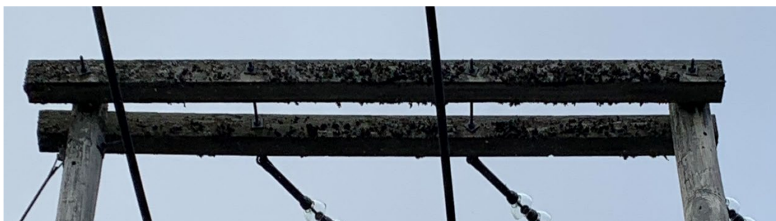
Figure C-2: Deteriorated 6.9 kV Wood Crossarms
