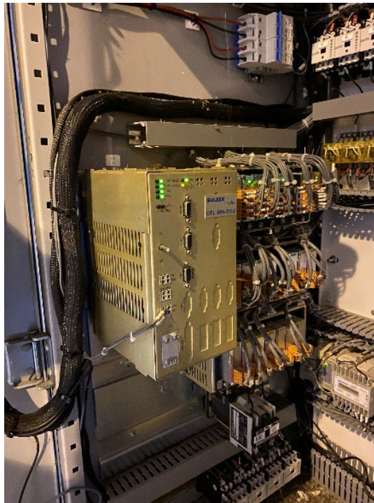
Figure 3 - Governor Control System Controller and Modules
