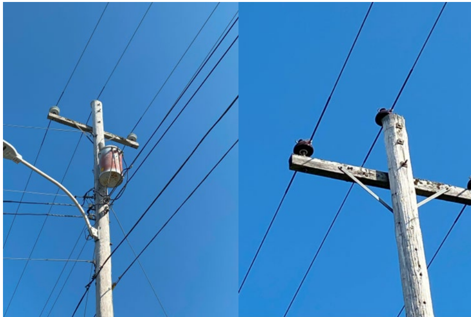
Figure 5 – Deteriorated Transformer and Insulators
