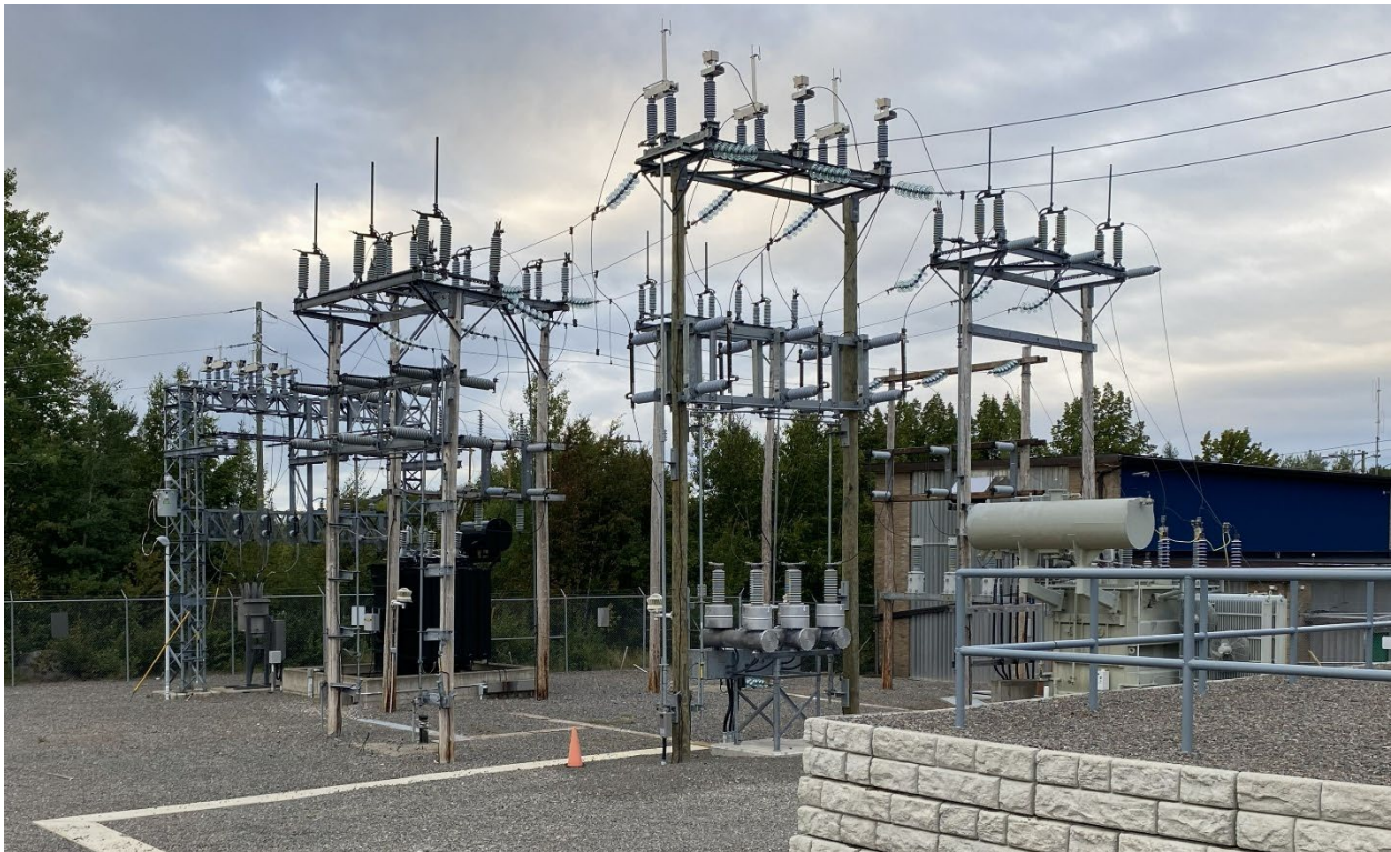
Figure B-1: RBK Substation
